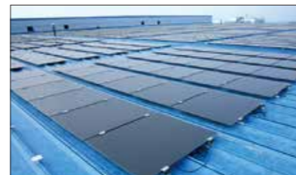
India, Roof Mount Systems-3MW
