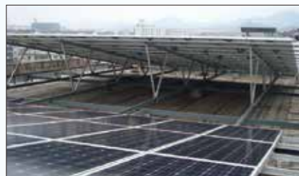
Jordan Flat Roof Mount-379.7KW
