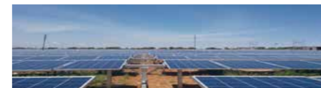
Horizontal single axis tracking system
