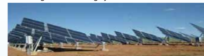
Double single axis tracking system
